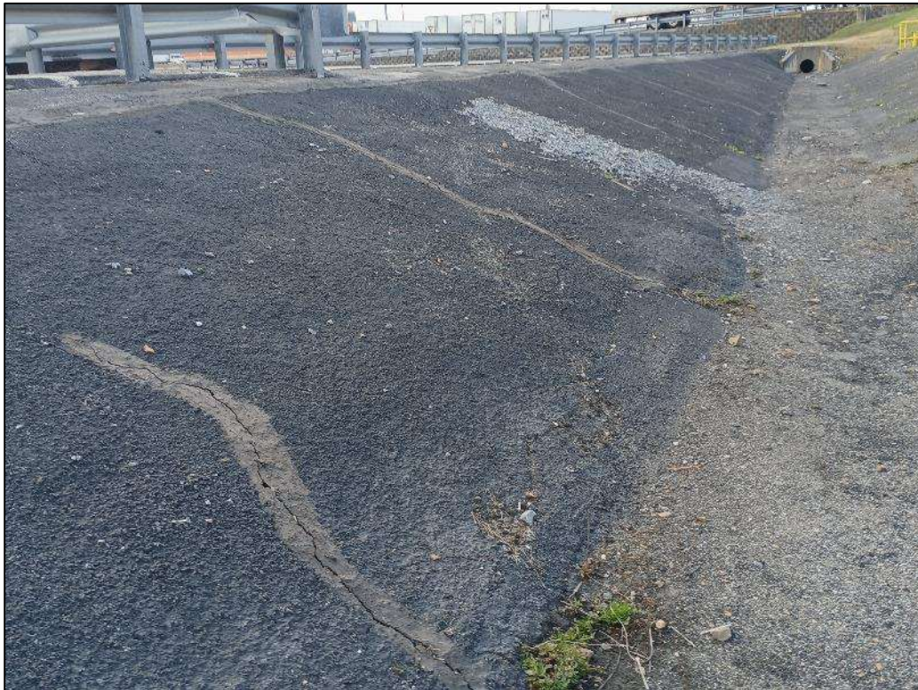
Photo looking south at cracks in the asphalt in the paved swale.
